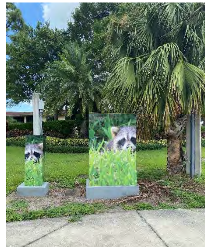
Figure 68: Utility Box Wraps at SE Walton Rd & Village Green Dr
