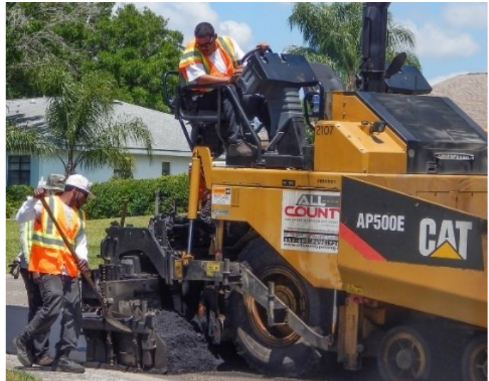
Repave deteriorated neighborhood streets (Source: Sun City Center, FL)
