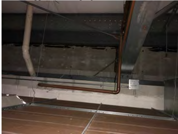
Photo: Copper Water Piping
