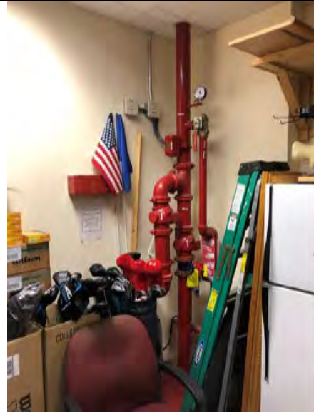
Photo: Fire Standpipe
