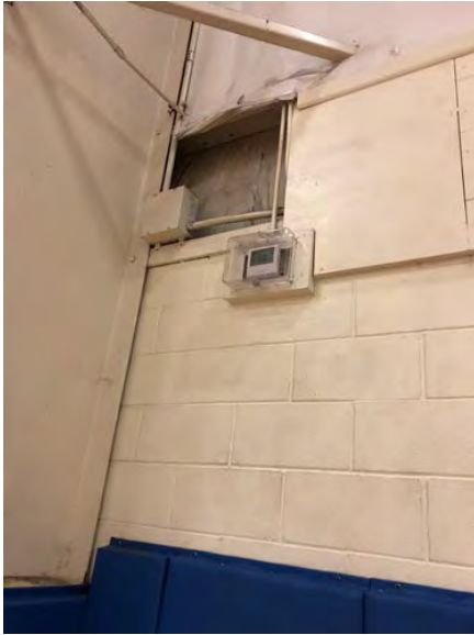
Photo: Gymnasium NE AHU - Thermostat
