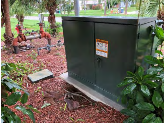
Photo: FPL Transformer #0-459-462-003
