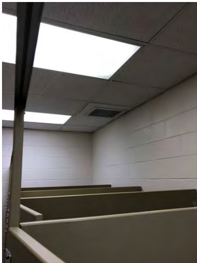
Photo: Men & Women Bathrooms Exhaust Fans
