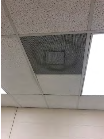
Photo: Lobby/Office - Supply/Return Grilles
