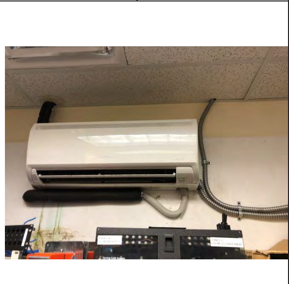
Photo: Mitsubishi Mini-split
