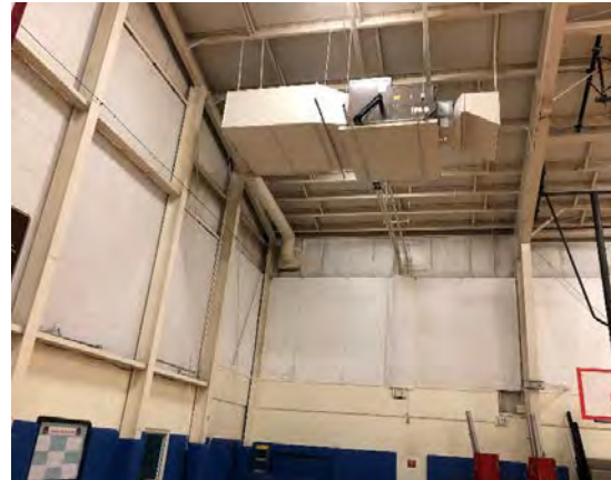
Photo: Gymnasium SW AHU – Supply/Return Grilles
