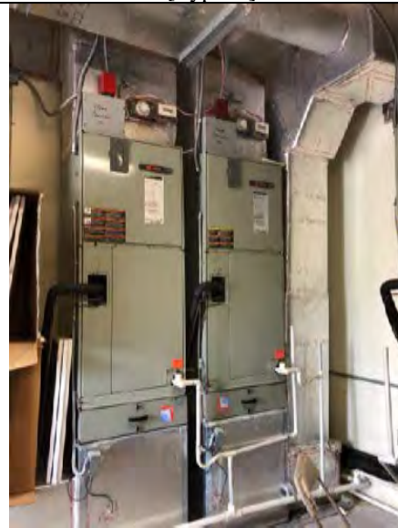
AHU-4A Trane [Typical]
