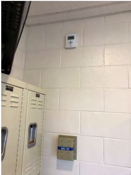
Photo: Lobby/Office A/C – Thermostat Missing Tamper Cover
