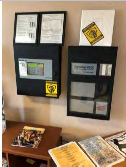
Photo: Fire Alarm Panel
