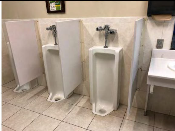
Photo: Flush Valve Urinal
