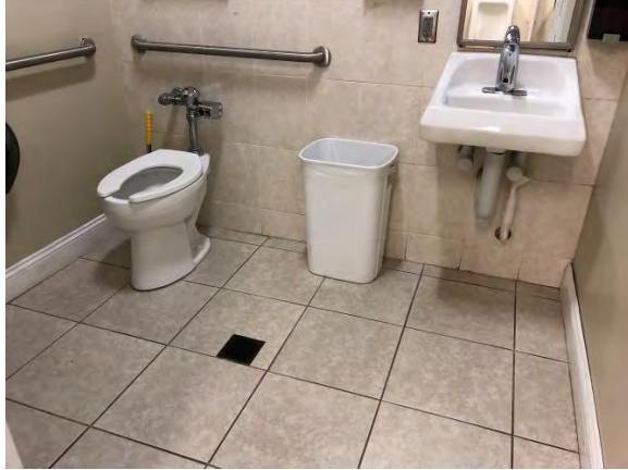
Photo: Flush Valve Water Closet
