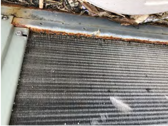
Photo: CU-7B Trane
