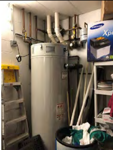
Photo: Gas Fired Water Heater
