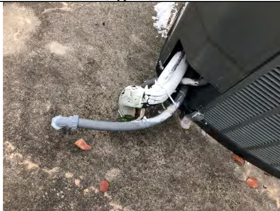
Photo: CU-1 Trane [Typical]
