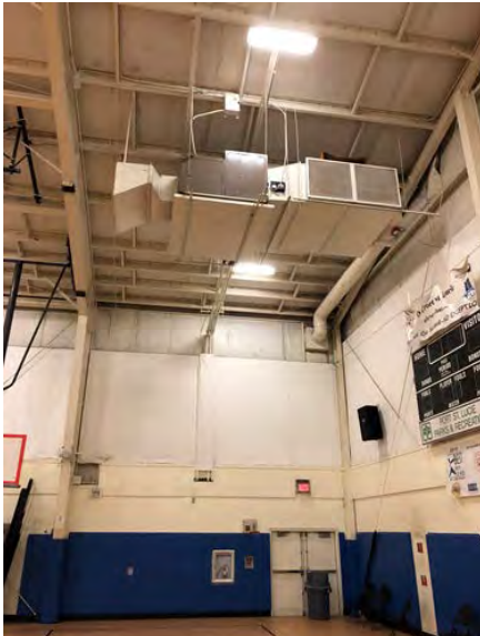
Photo: Gymnasium NW AHU – Sheet Metal Ductwork
