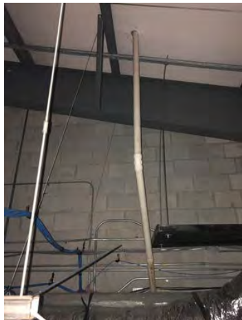
Photo: PVC Piping
