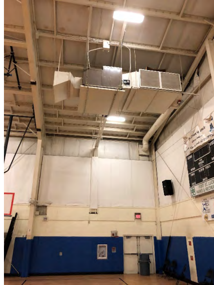
Photo: Gymnasium NW AHU – Thermostat Missing Protective Cover
