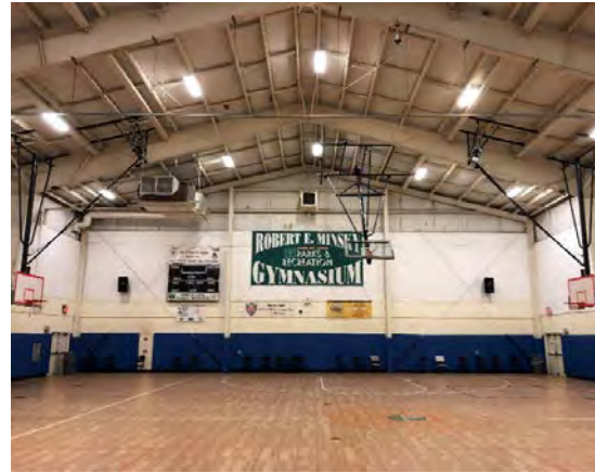
Photo: Gymnasium – 1x4 New LED Fixture
