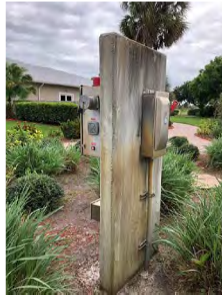
Photo: Exterior Site Lift Station
