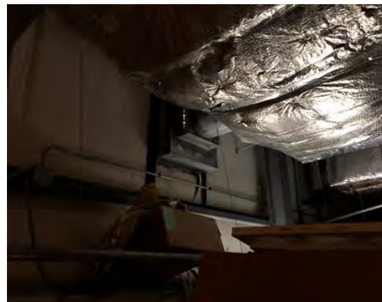
Photo: Gymnasium NE AHU – Return Air
