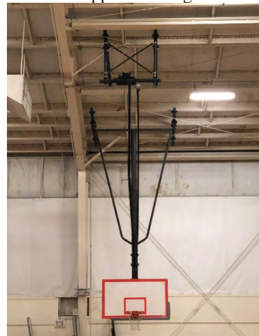
Photo 5.16: Basketball board equipment support framing
