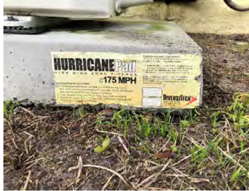
Photo 3.5: Mechanical equipment precast concrete pad
