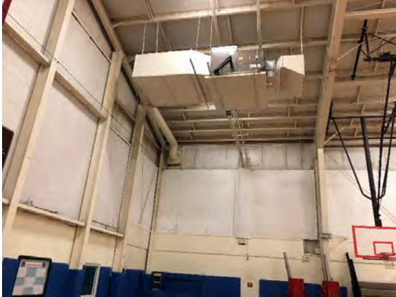
Photo: Gymnasium SW AHU – Sheet Metal Ductwork
