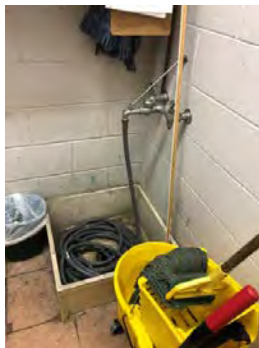
Photo: Janitor Sink
