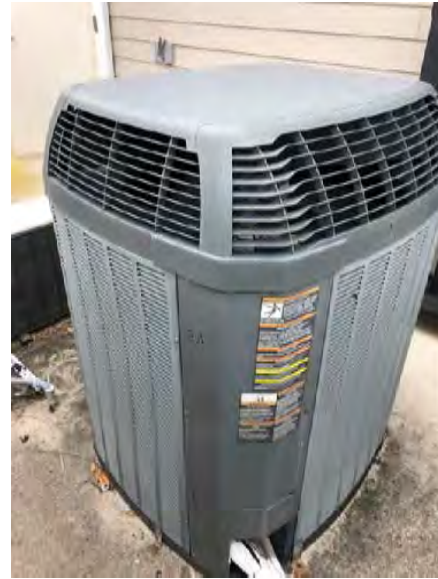
Photo: CU-1 Trane [Typical]
