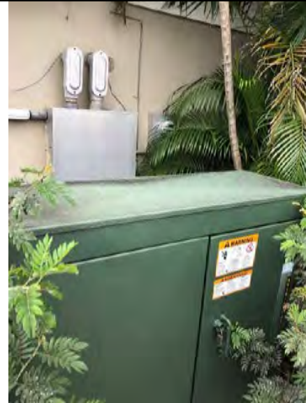
Photo: FPL Transformer # 66563381403
