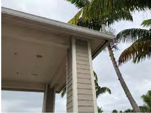
Photo 5.1: Steel beam with some surface rust at the front entrance port cochere
