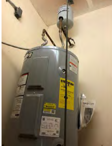
Photo: Electric Water Heater
