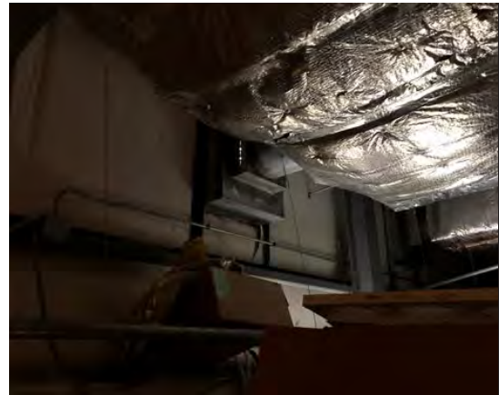
Photo: Gymnasium NE AHU – O/A Intake
