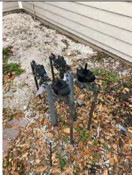
Photo: Cart Barn – Water Service
