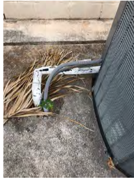
Photo: CU-4A Trane [Typical]
