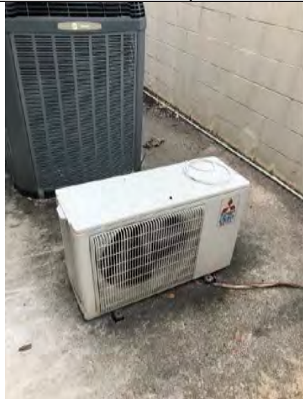
Photo: Mitsubishi Mini-split
