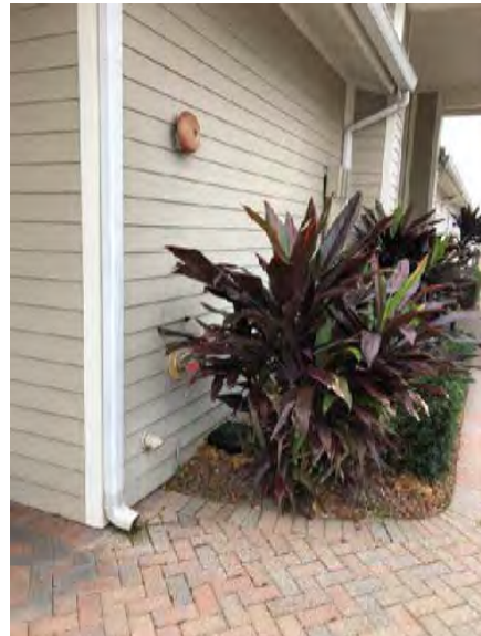
Photo: Fire Standpipe
