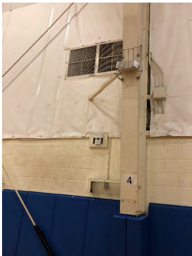
Photo: Gymnasium – Emergency Lights
