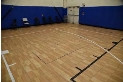
Photo 9.5: Gym flooring seam separation.
