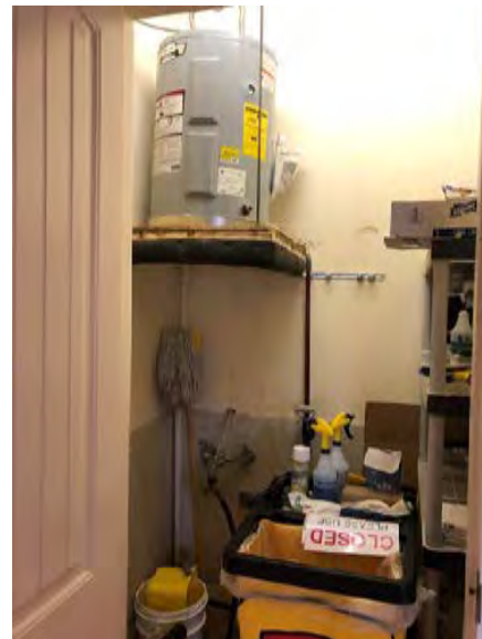
Photo: Electric Water Heater
