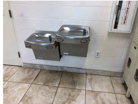
Photo: Drinking Fountains
