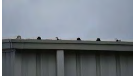
Photo 7.10: Open ends of the roof panels.
