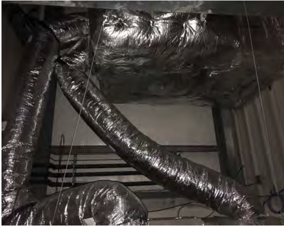
Photo: Gymnasium SE AHU - Sheet Metal Ductwork
