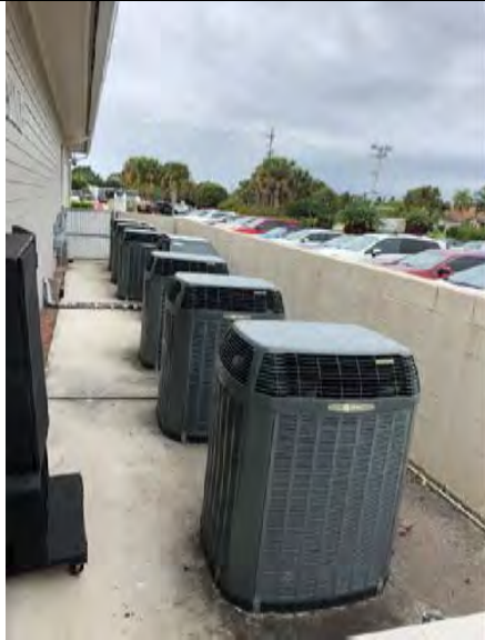
Photo: CU-1 Trane [Typical]
