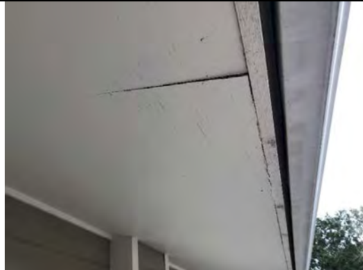
Photo 6.16: Partially detached exterior plywood ceiling panel
