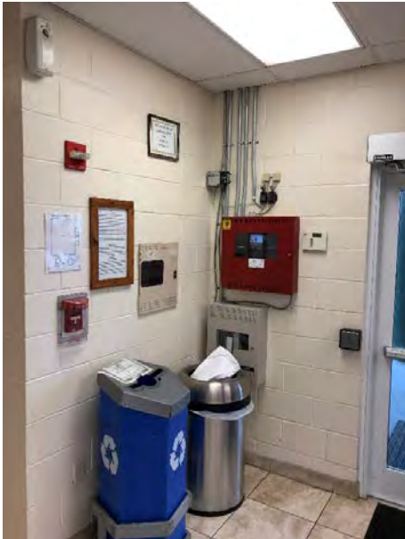
Photo: Fire Alarm Panel
