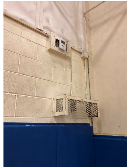
Photo: Gymnasium SE AHU – Thermostat Missing Protective Cover
