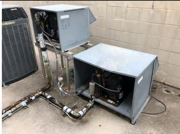
Photo: Kitchen Cooler/Freezer CU
