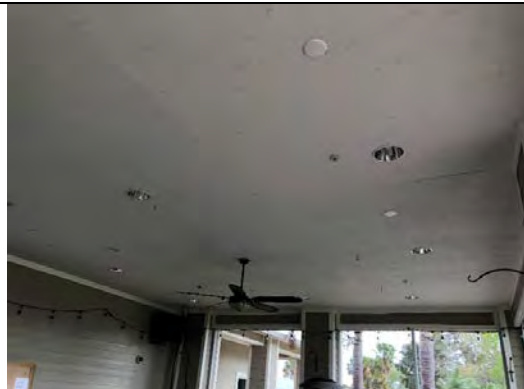
Photo 6.18: Unfinished joint and gaps between exterior plywood ceiling panels
