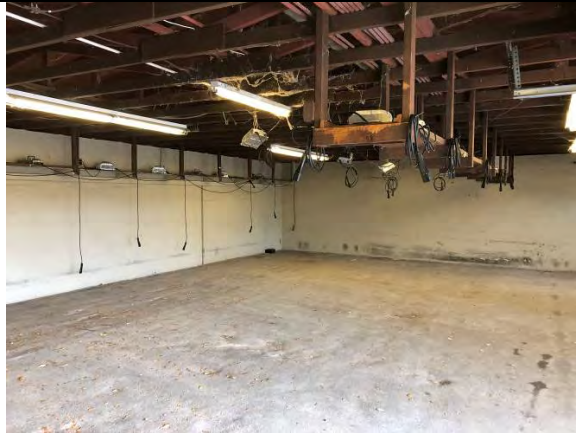
Photo: Battery Chargers
