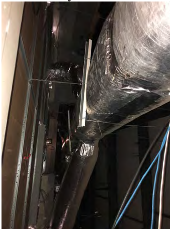
Photo: Lobby/Office - Sheet Metal Ductwork
