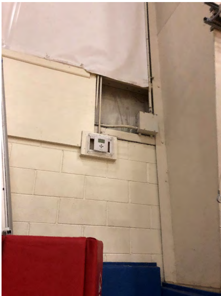
Photo: Gymnasium SW AHU – Thermostat Missing Protective Cover
