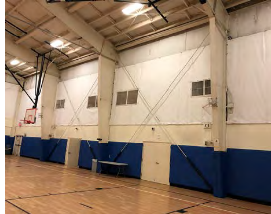
Photo: Gymnasium SE AHU – Supply Air Grille
