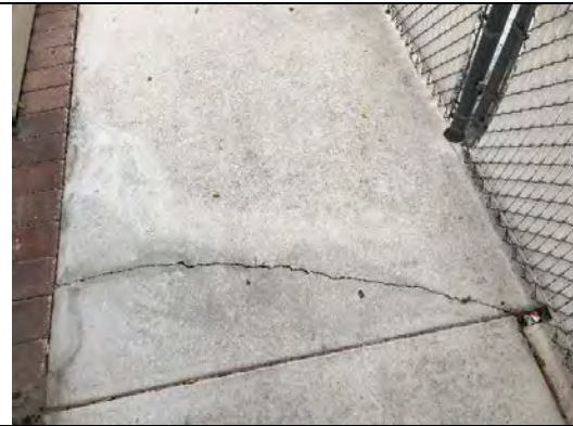
Photo 3.4: Cracked slab on grade section
