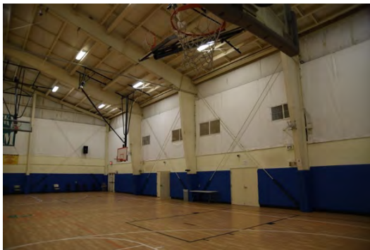
Photo 9.7: Structural steel has not been painted since the building was constructed.
