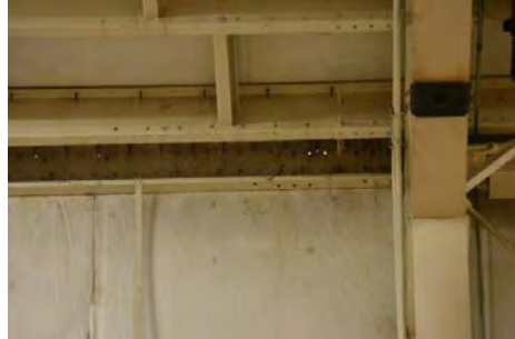
Photo 7.8: Daylight coming in through holes at the roof wall joint.
