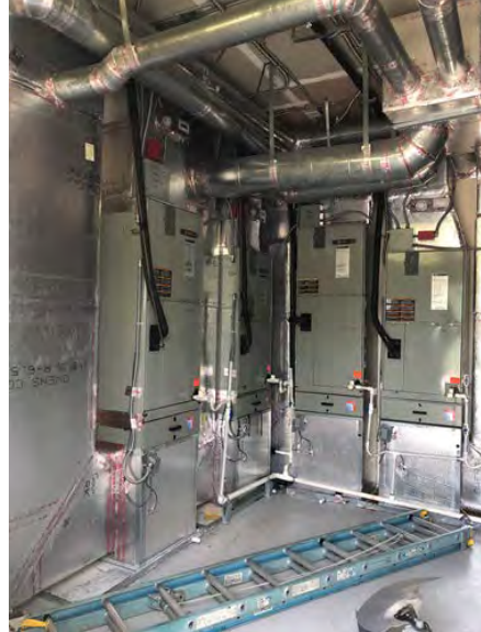
Photo: AHU-1 Trane [Typical]
