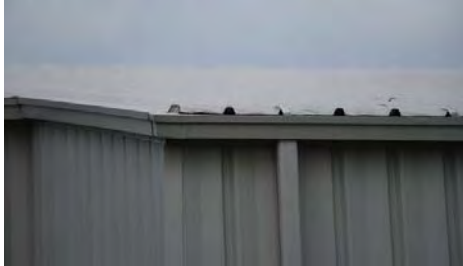
Photo 7.9: Open edges of the roof panels
