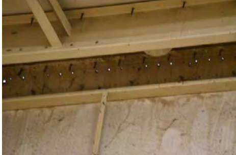
Photo 7.7: Daylight coming in through holes at the roof wall joint.
