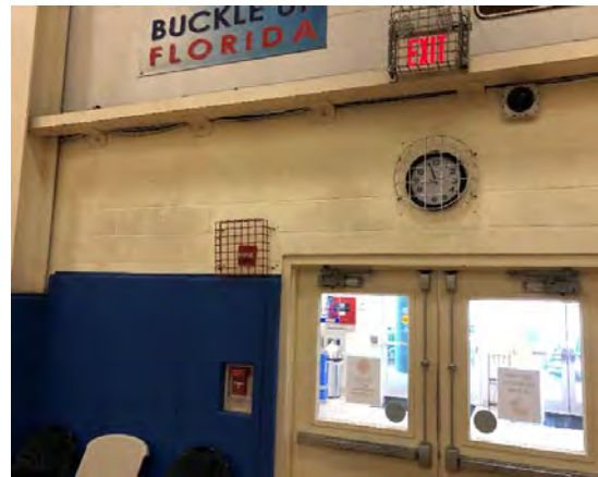
Photo: Gymnasium – Exit Lights
