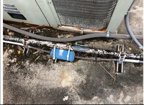
Photo: CU-7A Trane
