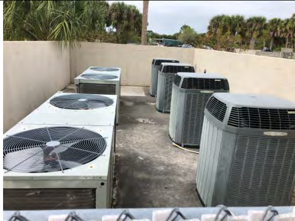
Photo: CU-4A Trane [Typical]
