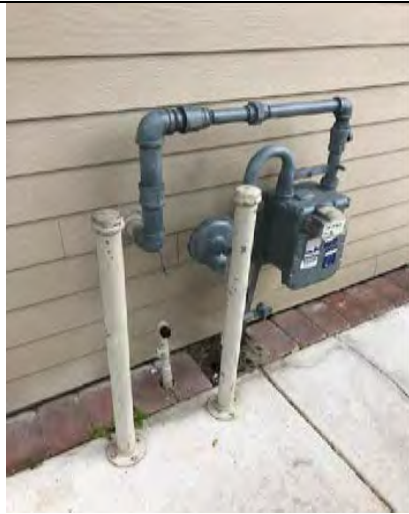
Photo: Natural Gas Meter
