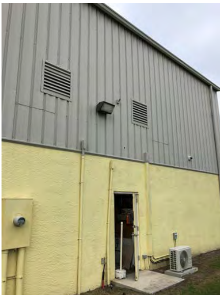
Photo: Gymnasium NE AHU – O/A Intake
