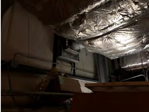
Photo: Gymnasium NE AHU – O/A Intake Ductwork
