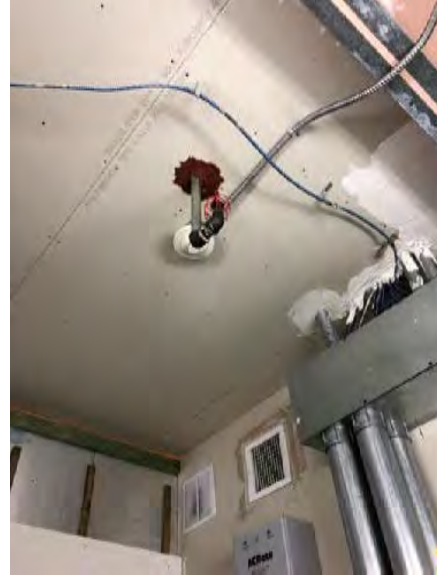
Photo: Smoke Detector
