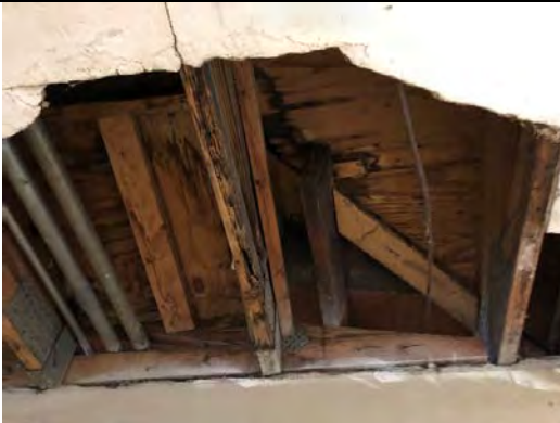
Photo 6.15: Decayed wood truss members and open ceiling in the golf cart building
