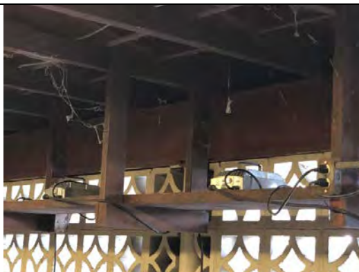
Photo 6.13: Golf Cart building Roof trusses and secondary wood framing and steel I beam with architectural block
