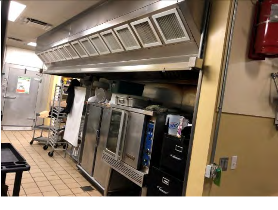
Photo: Kitchen Grease Hoods
