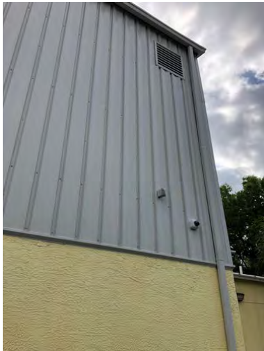
Photo: Gymnasium SW AHU – O/A Intake
