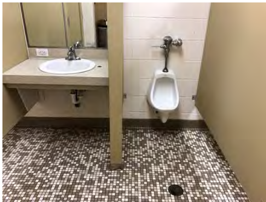
Photo: Flush Valve Urinal
