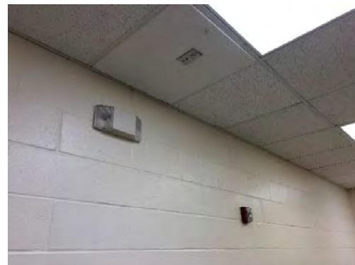
Photo: Lobby/Office – Emergency Lights
