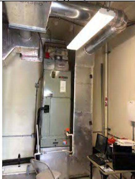
AHU-4A Trane [Typical]
