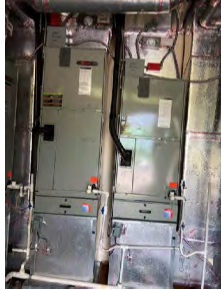
Photo: AHU-1 Trane [Typical]
