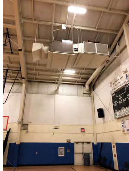
Photo: Gymnasium NW AHU – Supply/Return Grilles
