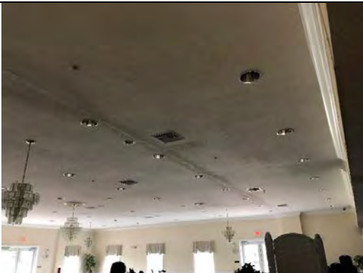
Photo 6.17: Cracked ceiling due to girder truss deflection and movement in the truss to girder truss connection
