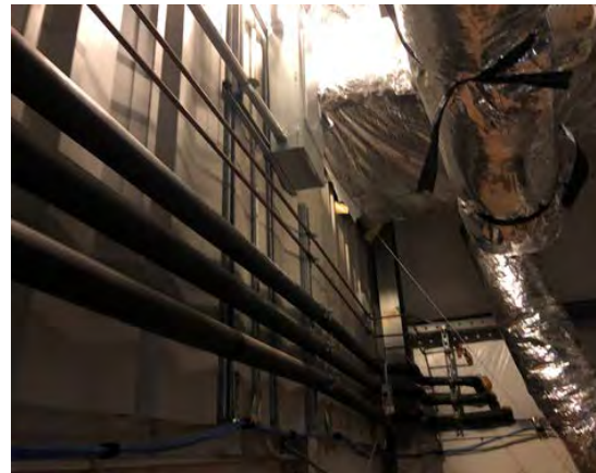
Photo: Gymnasium NE AHU – Sheet Metal Ductwork
