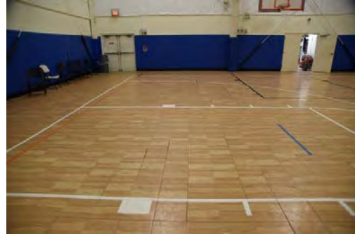
Photo 9.6: Gym flooring seam separation.
