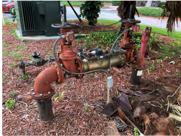
Photo: Fire Service Backflow
