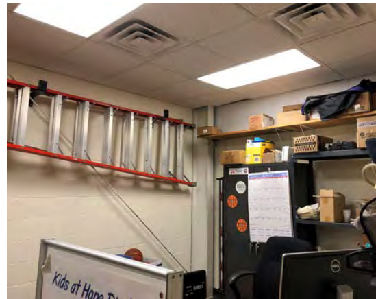
Photo: Lobby/Office - Supply/Return Grilles
