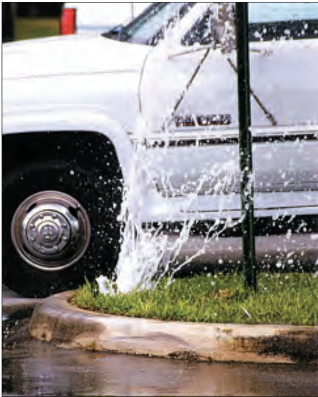
Figure 11. Water gushing from broken head.
