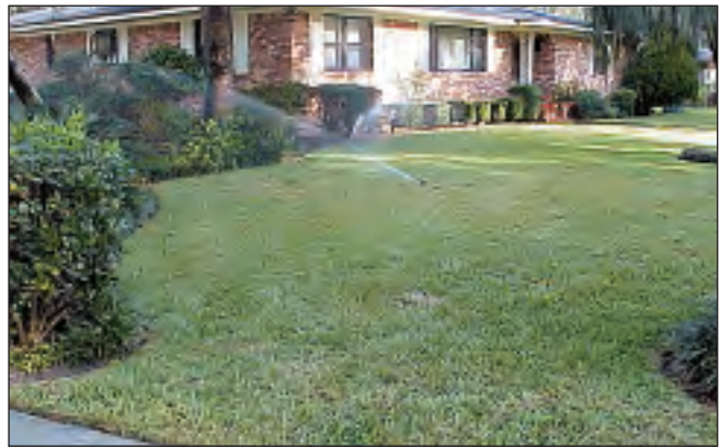
Figure 8. Poor design; system does not match irrigation requirements. The area needs to be rezoned with landscape and turf separated.
