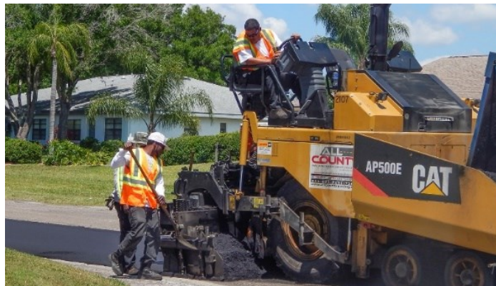
Repave deteriorated neighborhood streets (Source: Sun City Center, FL)
