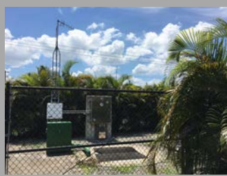
Wastewater lift station
